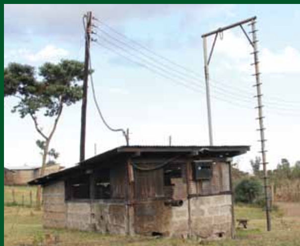
Ndibithi borehole pump house
