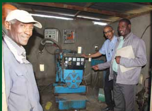
Inspecting generator unit at Shamba Boy borehole
